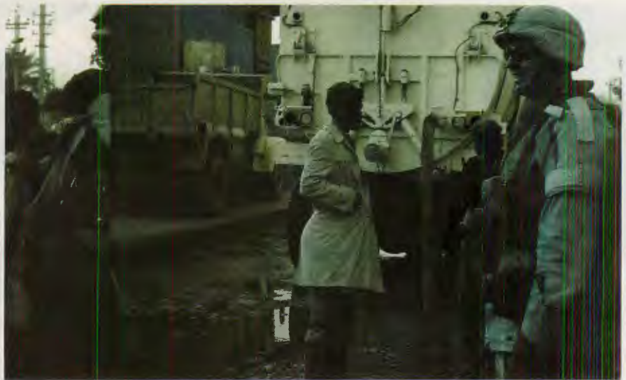
Capt. Douglas Chapman, Co. B, 1-12 Cav, works with contractors to remove sewage from the streets of Sadr City. Under Saddam, this slum was known as Saddam City and suffered severe neglect to its infrastructure. U.S. Army Photo by Capt. Michael Martinez
